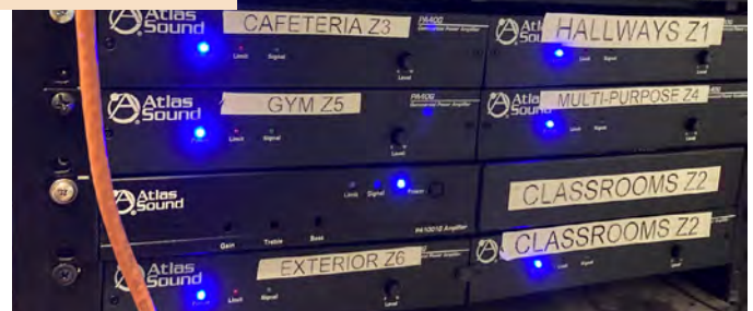
Public Address (PA) headends (controllers) installed in an IT equipment rack in a Telecom Room. These headends can be programmed to trigger actions based on specific events.
