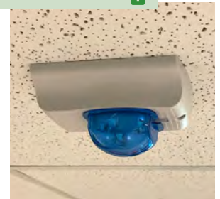
An interior ceiling-mounted blue light.
